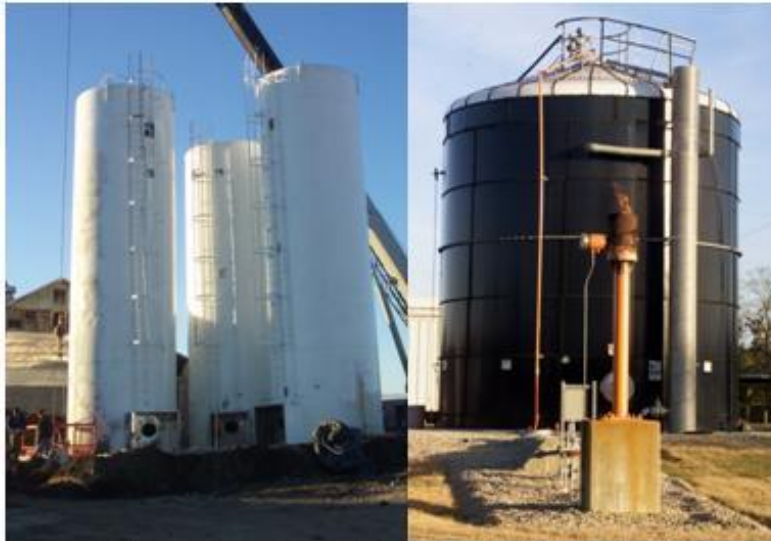
Anaerobic Sludge Blanket Attached Media
